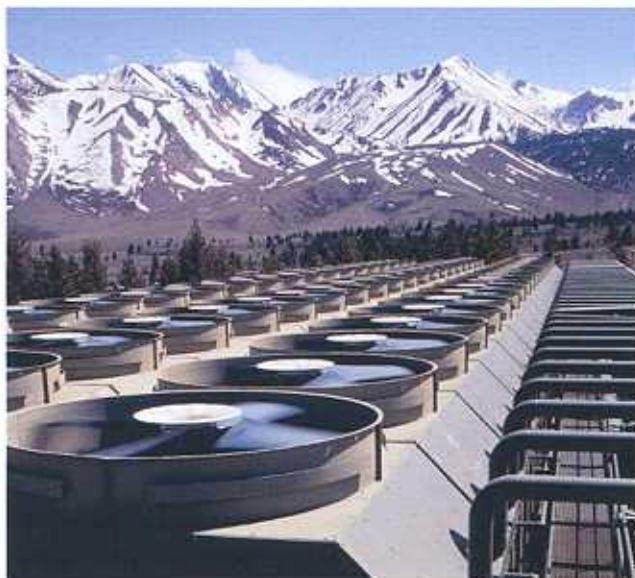
Mammoth-Pacific's fin fan condensing system relies on air cooling, but performance—and power output—suffer during the hot summer months.
