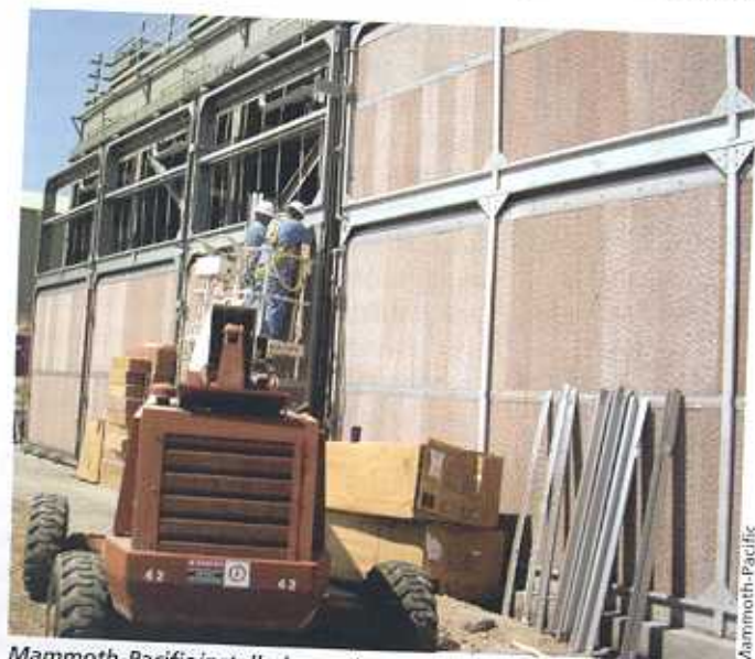
Mammoth-Pacific installed experimental evaporative cooling systems last year, boosting power production as much as 20 percent.
